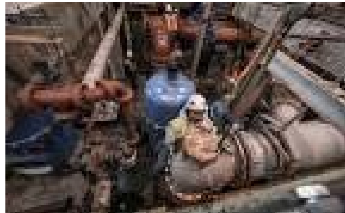
Wastewater systems under pressure
